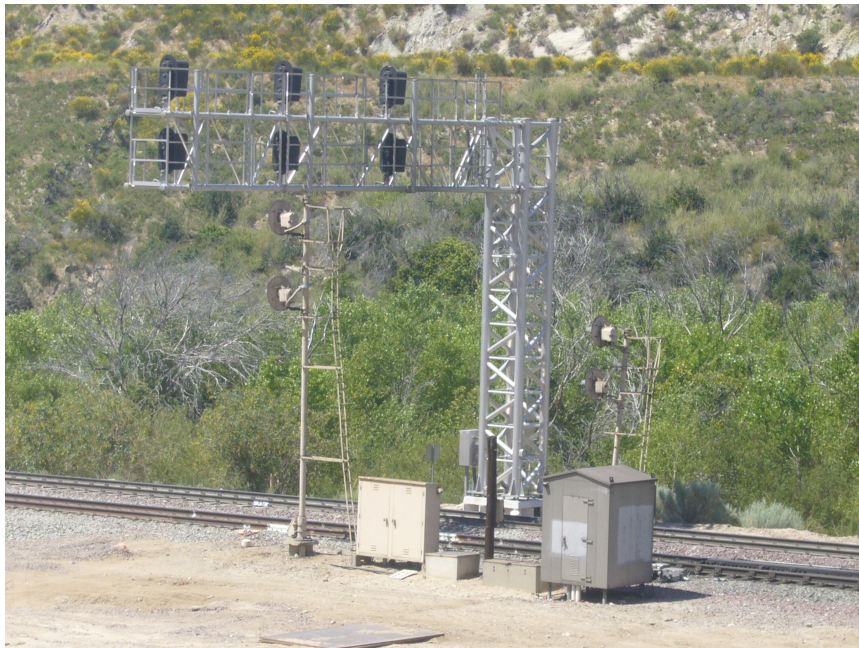
Protecting the new crossovers at the west end of Cajon is this new cantilevered three-track signal bridge. Note the soon-to-be-removed, old ATSF signals under the span. Photo by Dennis White.
