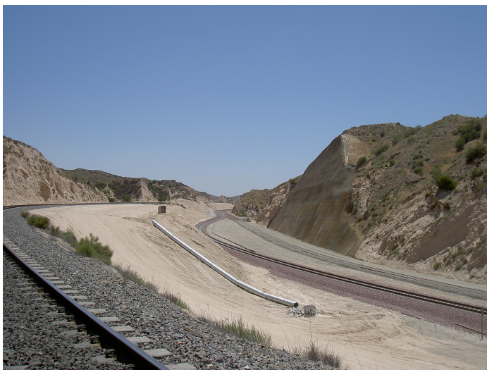
Alray's Tunnel 2 is gone and all the rubble cleaned up, but the shoofly around the demolition site remains. Note the "Keystone" monument on the embankment near the upper end of the drainage pipe. Photo by Jack Barich.
