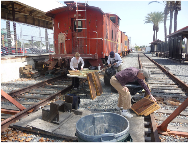
Stephanie White, Harold Benash and Jack Barich strip old foam from caboose benches preparatory to installing new upholstery. Photo by Dennis White
