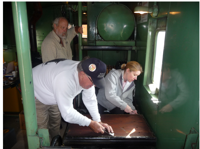
Stephanie White and Harold Benash dig out old tacks while Dave Norris supervises preparatory to installing new upholstery. Photo by Dennis White
