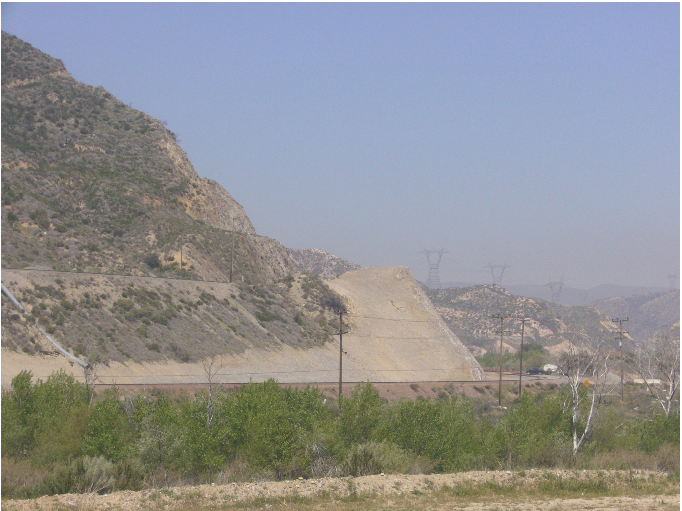
The cut at Swarthout Canyon required six months of blasting and grading to make room for the new third track through Cajon Pass. The Union Pacific (ex Southern Pacific) Colton Cut-off is visible at near the top of the cut. The trees at the bottom of the photo mark the location of Cajon Creek and the "low water bridge" of Swarthout Canyon Road.
